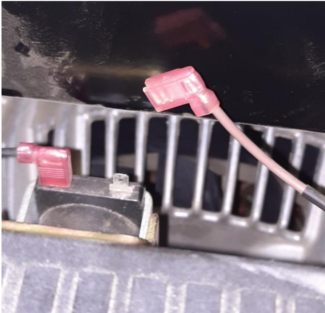
Figure 3 - Disconnected solenoid power cable
